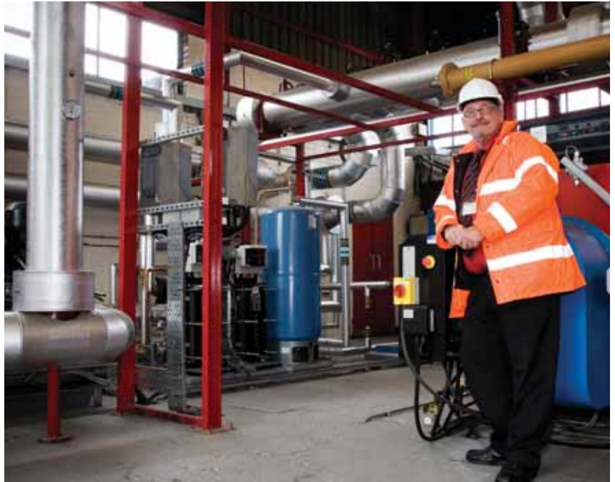
Wrightington Wigan and Leigh's new boiler house has made a huge difference to the trust's overall footprint
